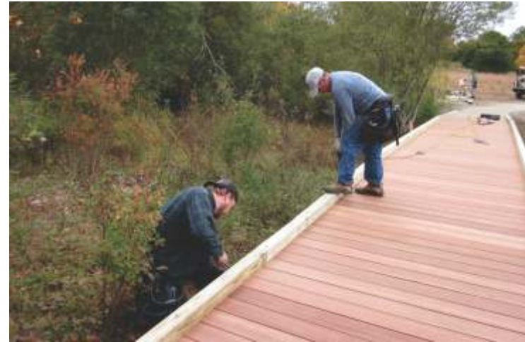
Workers from Brown Building Company put the finishing touches on the boardwalk.
