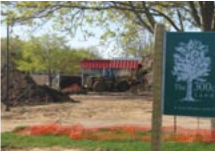
Work is underway to amend the soil for the upcoming streetscape plantings at Teaticket Park.
